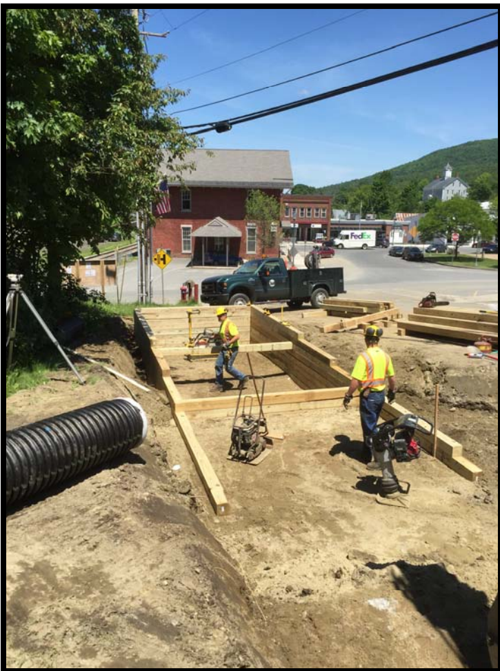
This bioretention area on Central Street will catch runoff from the drainage areas of two catch basins.
